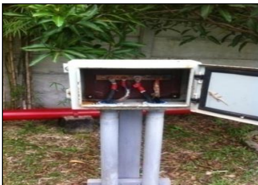
Gamabar 4.4 Junction Box
